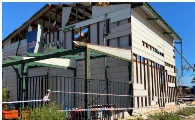
Asbestos materials found in Kalbarri, post Cyclone Seroja.
