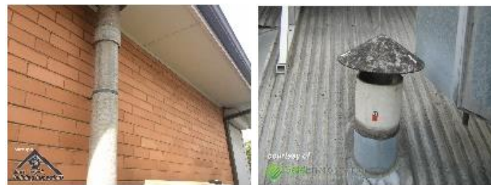
Flue pipes and fittings.
